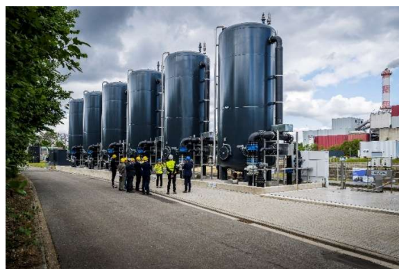
Flanders first advanced wastewater treatment plant for micropollutant removal from urban wastewater in Aartselaar.
